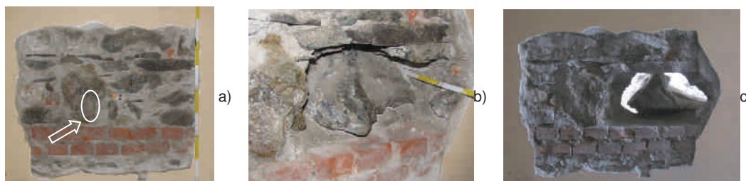
Figure 4: Inspection HSP- I5-6 at the first floor: three phases of the removal of a large stone used as “diatono”.
